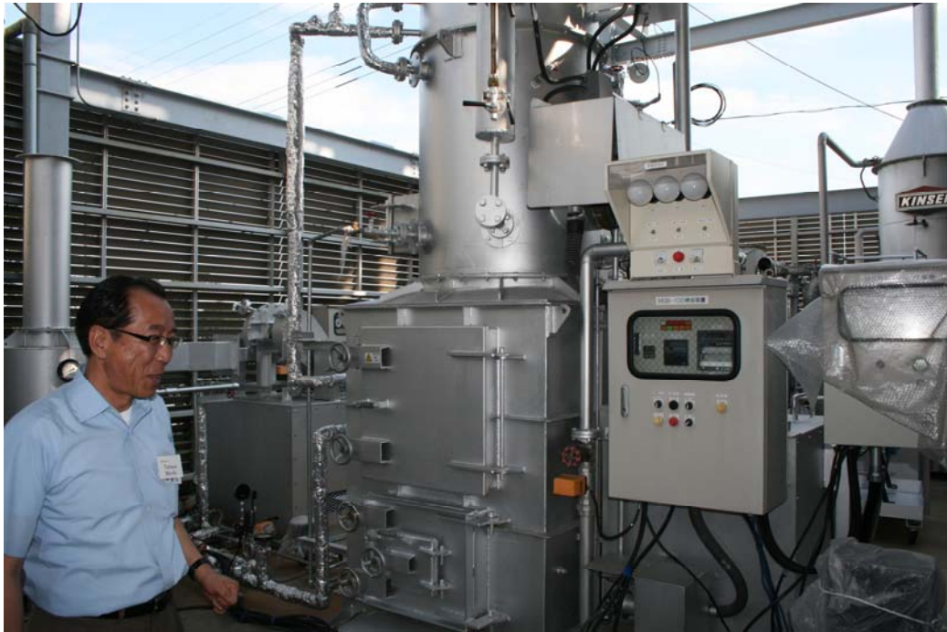
Figure 11: A Kinsei Sangyo Company Gasification System
