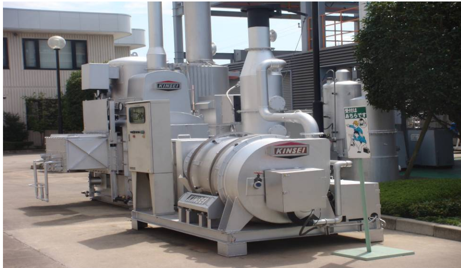
Figure 2: Kinsei Gasification System in Japan 4
