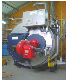
Waste Heat Boiler
